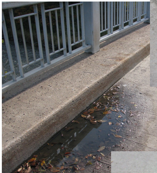
Below: Ponding on deck associated with plugged deck drain.
