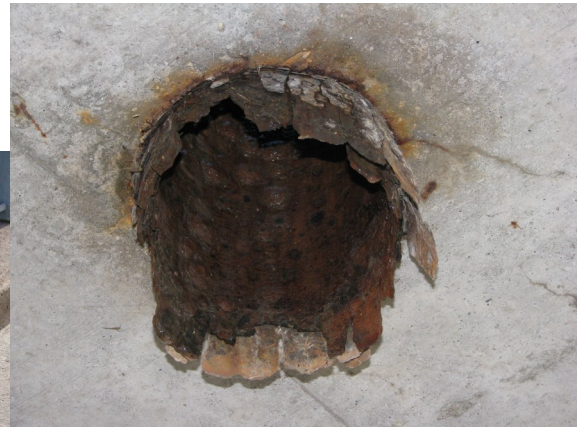
Above: Severely corroded deck drain requiring replacement.
