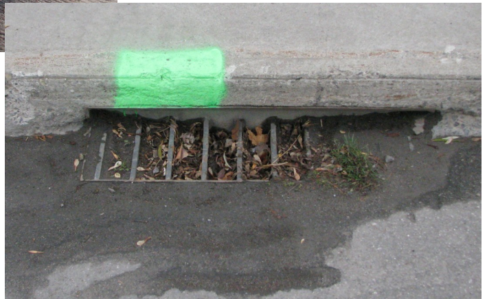
Right: Poorly maintained deck scupper. Ideally drains should be cleaned spring and fall.
