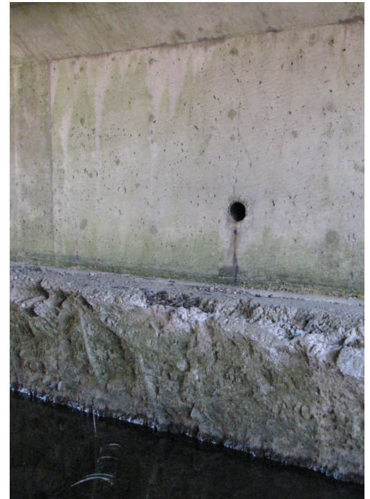
An otherwise good open-footing rigid frame concrete culvert where the foundations have been compromised by channel lowering to suit agricultural land drainage.
