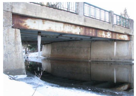
Example of a bridge near Kingston, ON where rehabilitation now or replacement later is not obvious.
