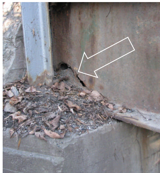
Perforated girder end resulting from lack of cleanliness.
