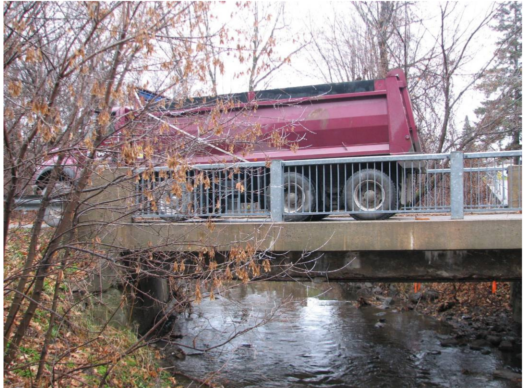
Picture above is of partly loaded tri-axle truck utilized for load testing Elm Street Bridge
