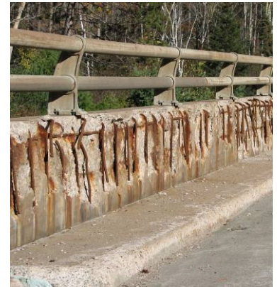
Severe spalling Damage to a parapet wall on a bridge on Hwy 17. The tarnishing of the railings can be characterized as a slight Defect.
